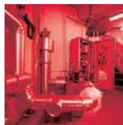
■ Air conditioning units
